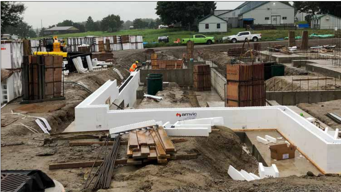
Construction on the new peopleCare long-term care home is well underway and expected to open on time next year.
